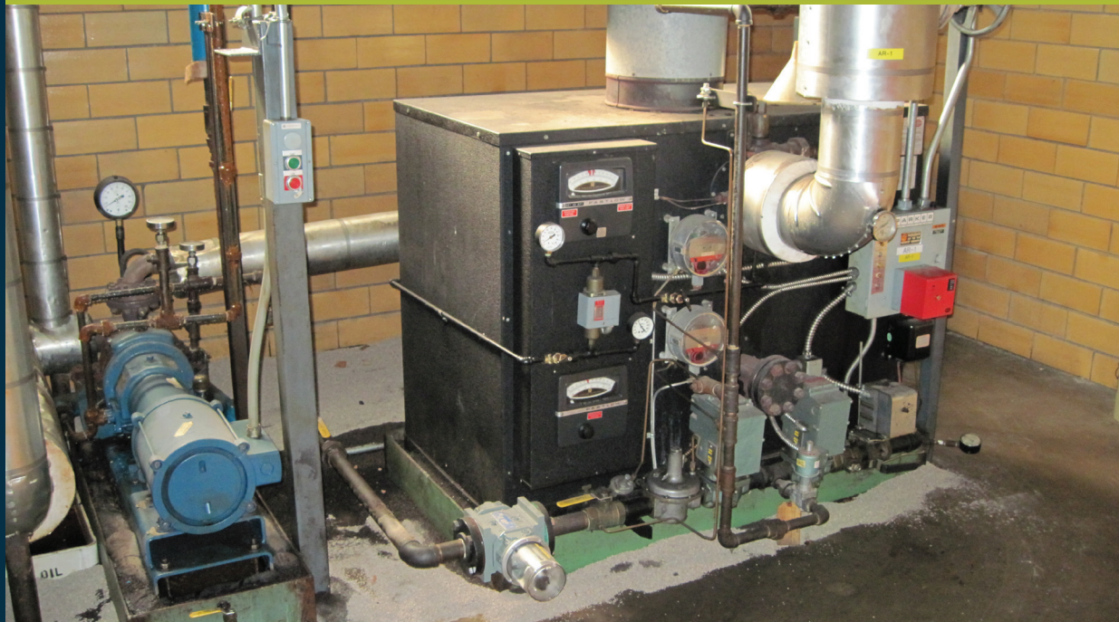
Parker Boiler HT1008 industrial high temperature thermal liquid heater at Worlds Finest Chocolate.
